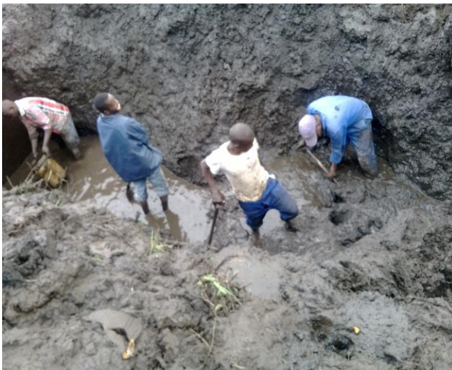
7C: Search for a burst pipe in Limbe Zone
