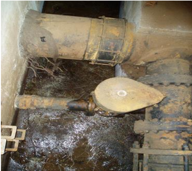
7A: Leaking old transmission main at Walkers Ferry
