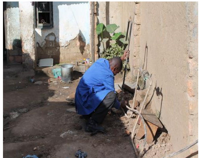
7D: BWB Plumber uprooting (meter bypass) Illegal connection in Ndirande Township
