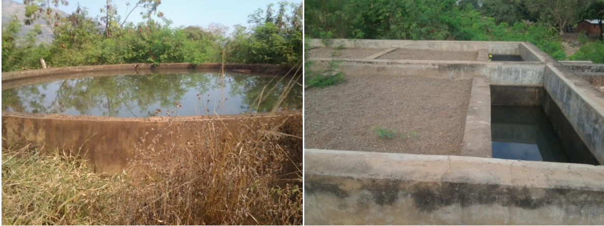
Figure 14: Sedimentation Tank (on the left) and Slow Sand Filters (on the right) in EBWSS
