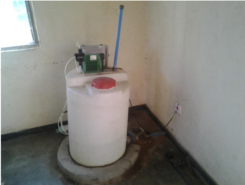
Figure 9: Chlorine Dosing Equipment at MFWSS
