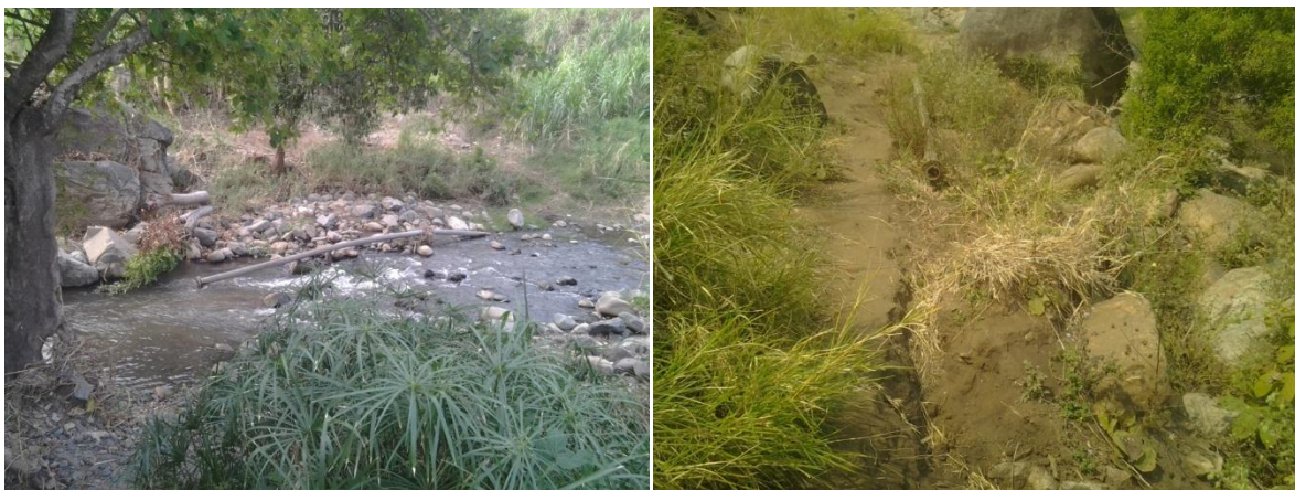
Figure 21: Theft and Vandalism of Transmission Pipelines in EBWSS
