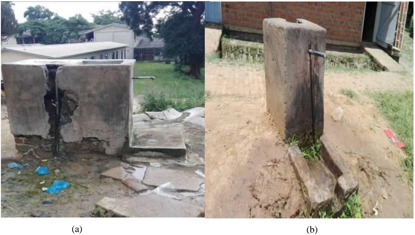
Figure 1: Condition of water access points in some secondary schools in Blantyre City
