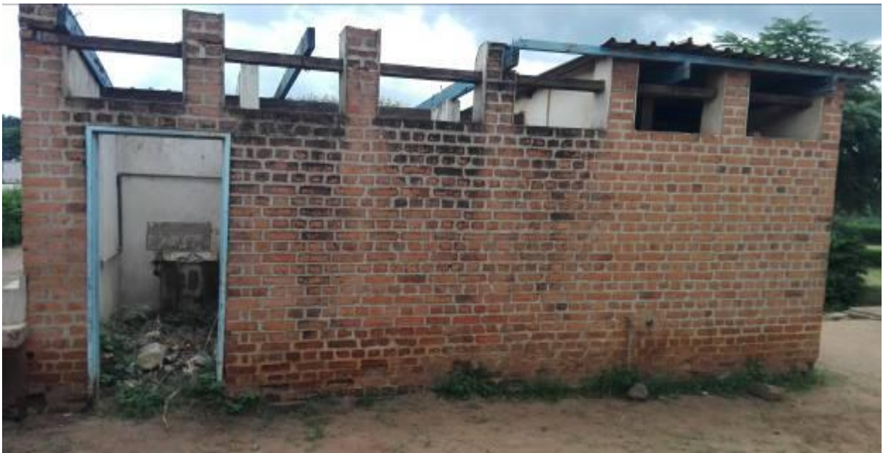
Figure 6: blocked and vandalised toilet for boys in one of the school premises
