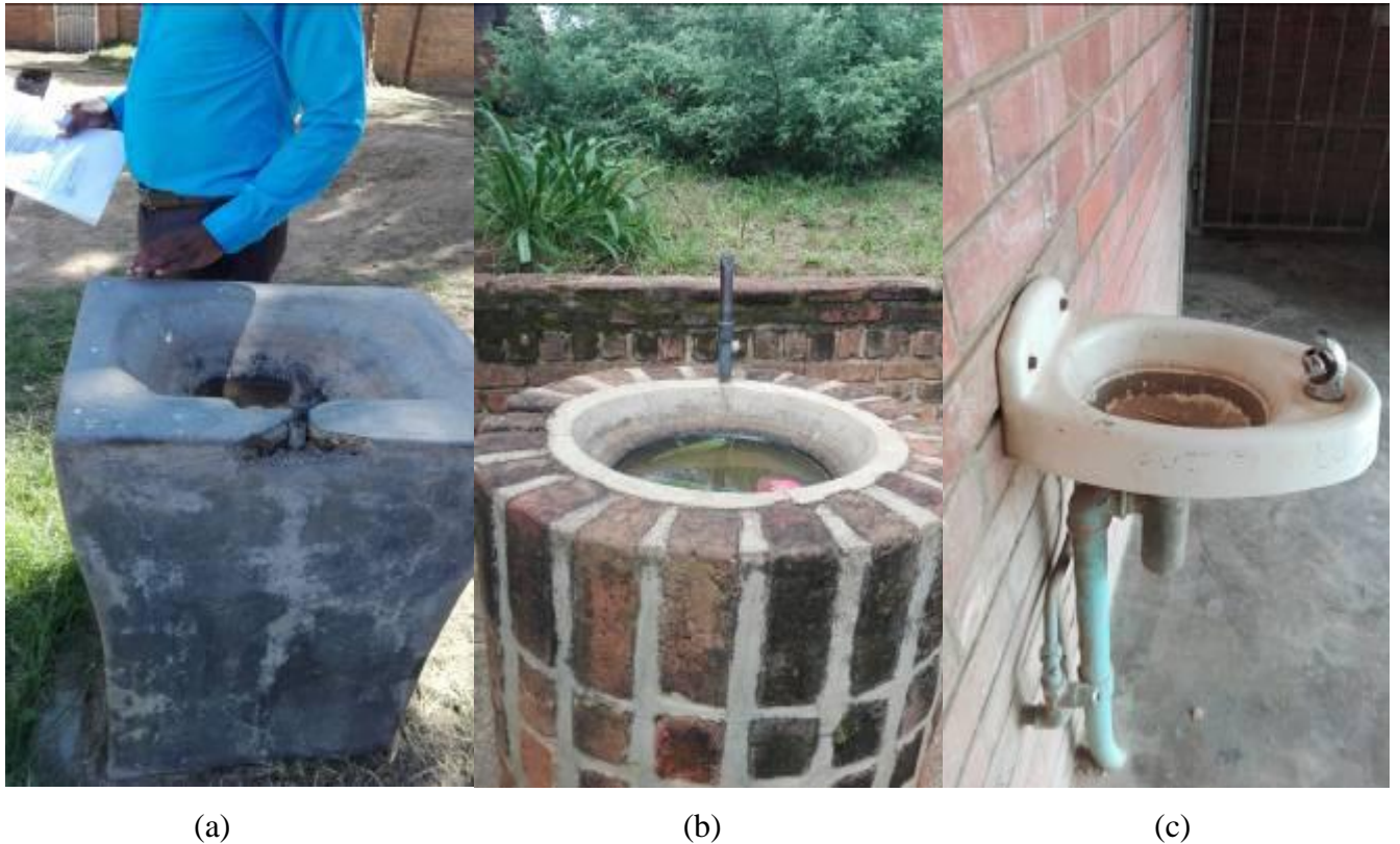
Figure 4: Abandoned water access points in some secondary schools in Blantyre City
