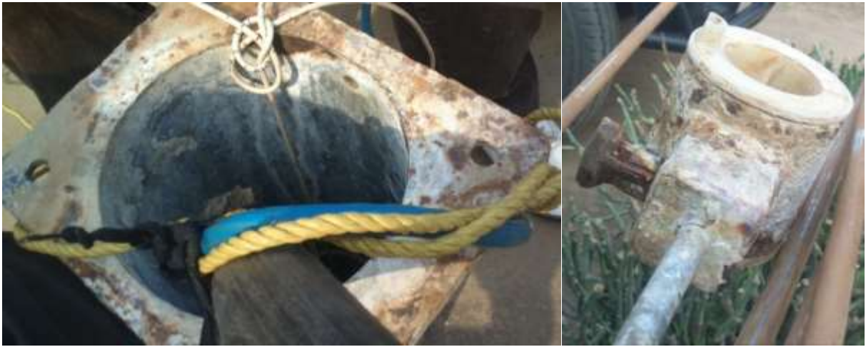
Figure 16: Severe Corrosion Due to Salty Water
