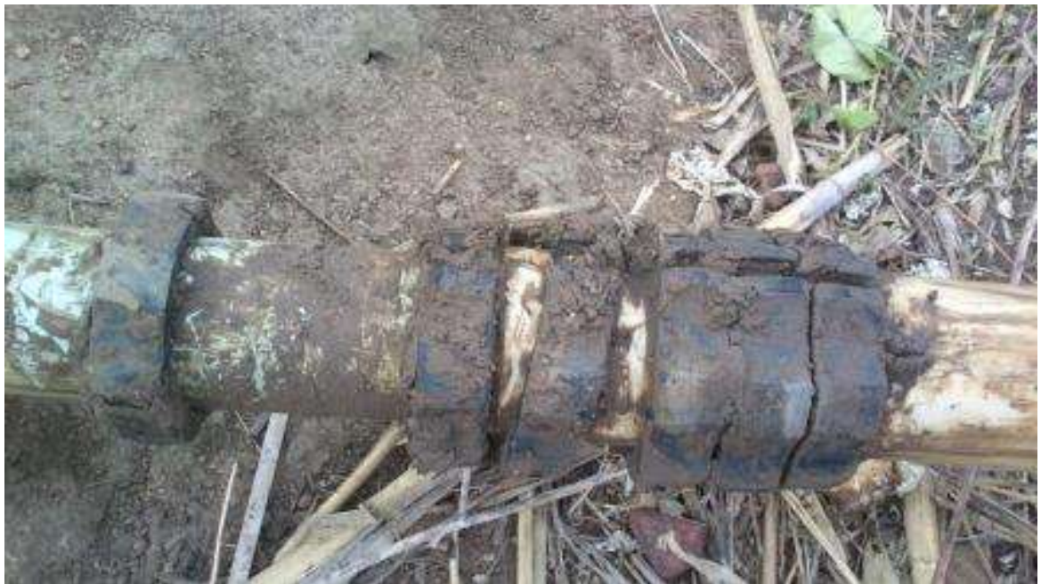
Figure 17: Termite Mound Developing in a Borehole (Top Picture) and Muddy Rising Main (Bottom Picture)
