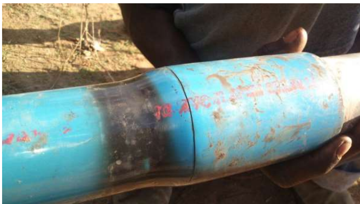
Figure 15: Cracked Rising Main
