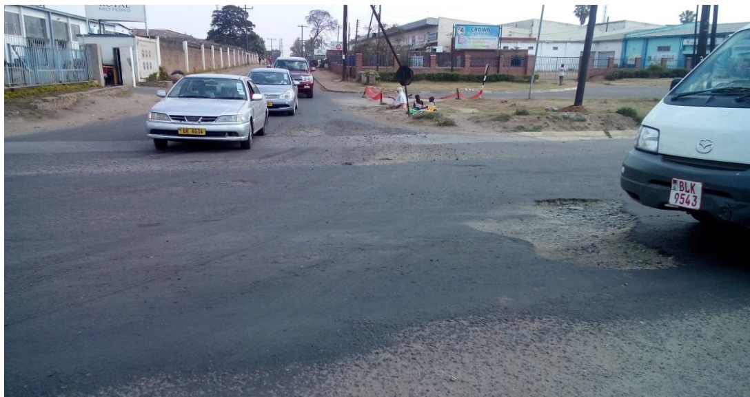
Figure 3.2: Potholes on Newly Constructed Blantyre-Zomba Road
