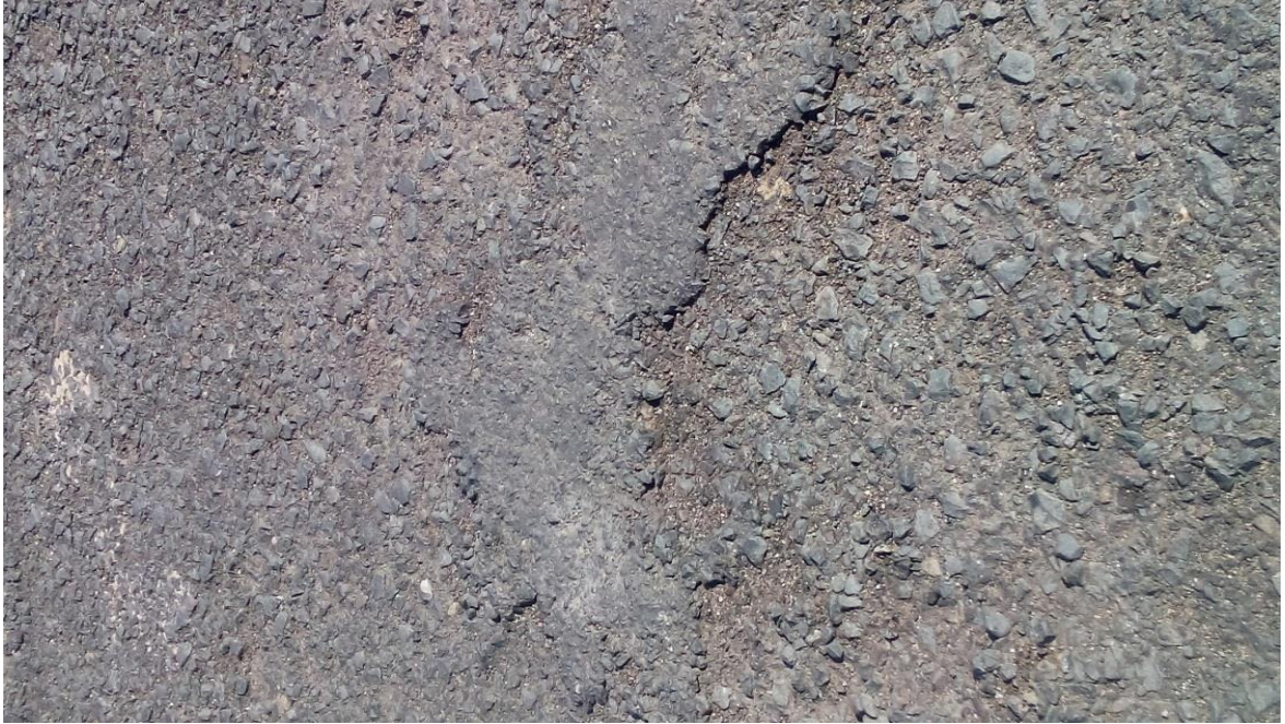
Figure 2.3: Surface Defect Due to Loss of Chippings
