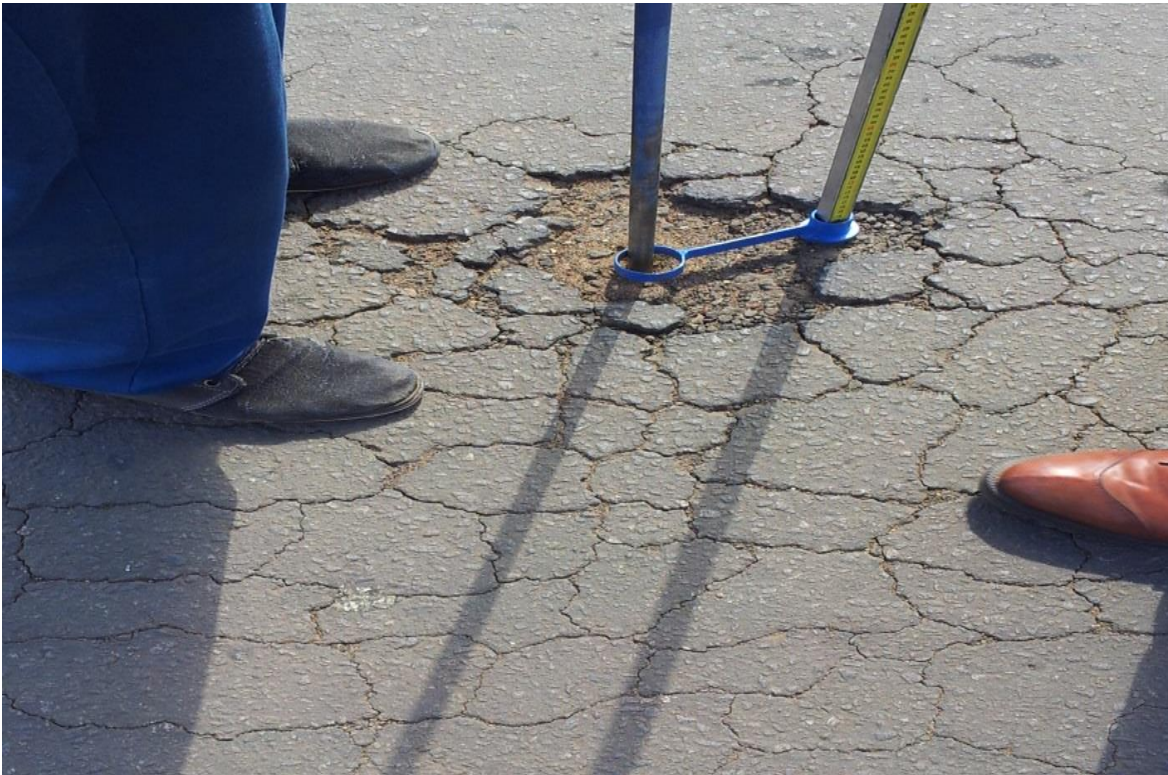
Figure 3.3: Heavily Cracked Mugabe Highway
